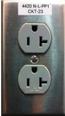
An example of a label on an outlet.
